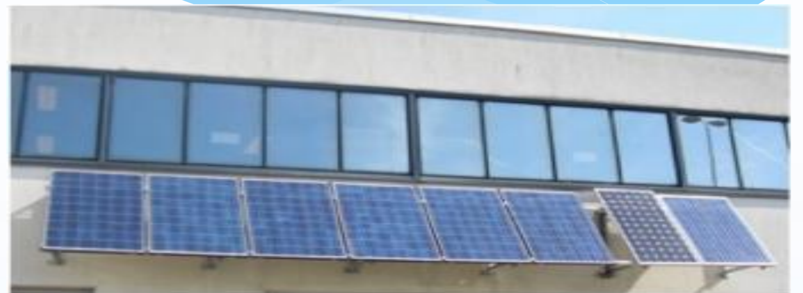
Figure 3: Photovoltaic (PV) Polycrystalline modules.
